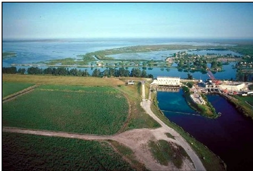
S-2 pumping station on the south end of Lake Okeechobee. (Source: South Florida Water Management District.)
